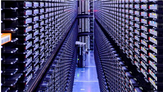
Network Infrastructure & Data Centers
